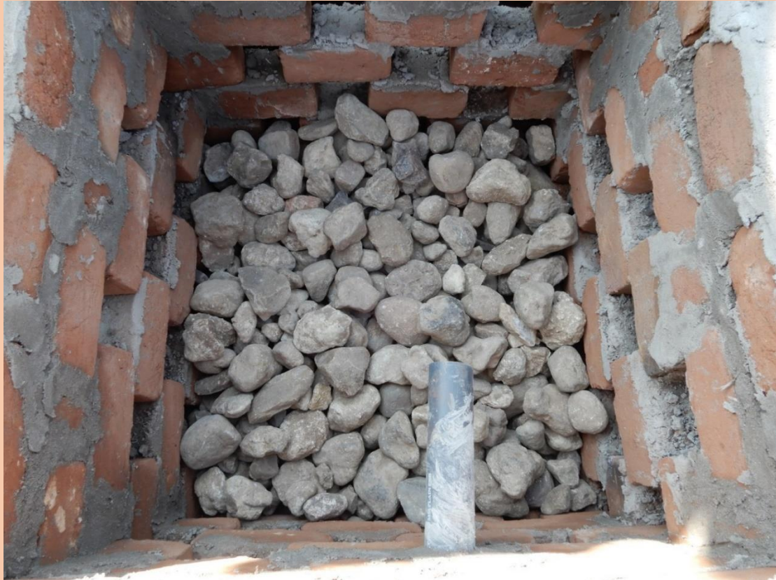
Soak pit developed near handpump in district Hoshangabad, state of Madhya Pradesh (Photo: FH India)
